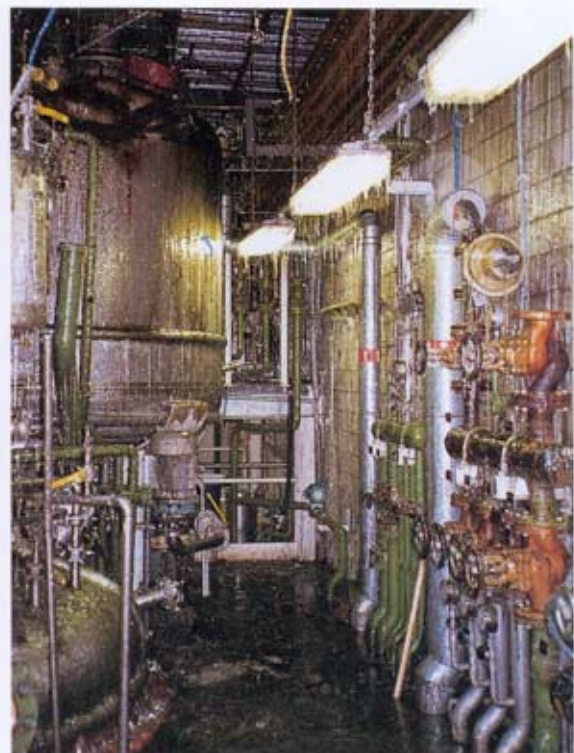
Within a radius of 15 metres all plant parts were contaminated with adhesive.
